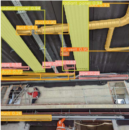
Figure 10: Failure case: Overwhelming density of parallel pipes and conduits. High overlap leads to instances being merged by NMS or parts of elements being missed.
